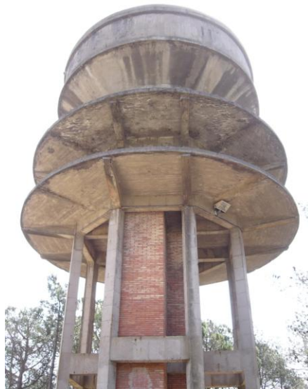
Figure 3. Reclaimed water storage tank at Lloret de Mar.
