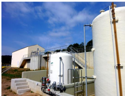
Figure 1. General view of the water reclamation plant of Lloret de Mar.
